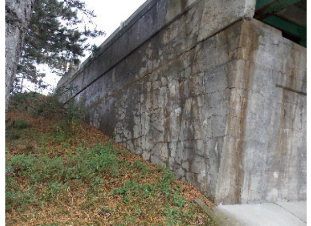
ASR Damage on Bridge #1563 Abutment
