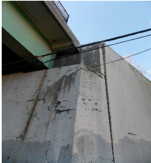
ASR Damage on Bridge #5799
