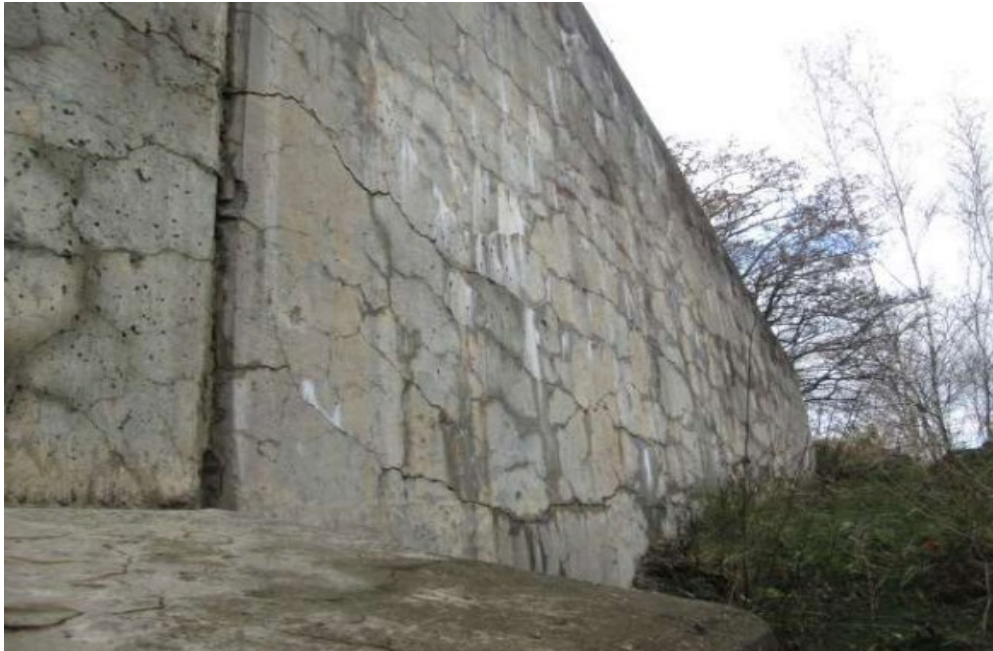
ASR Damage on a Bridge #1562 Wingwall
