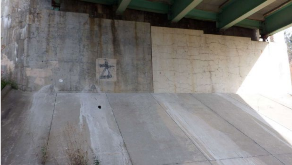
Extensive ASR Damage on Bridge #1560
