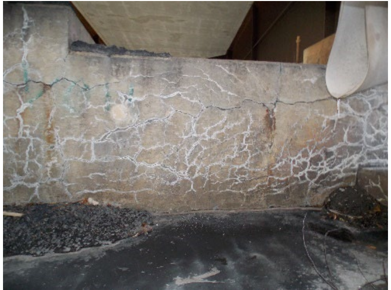
ASR Damage on Bridge #1558
